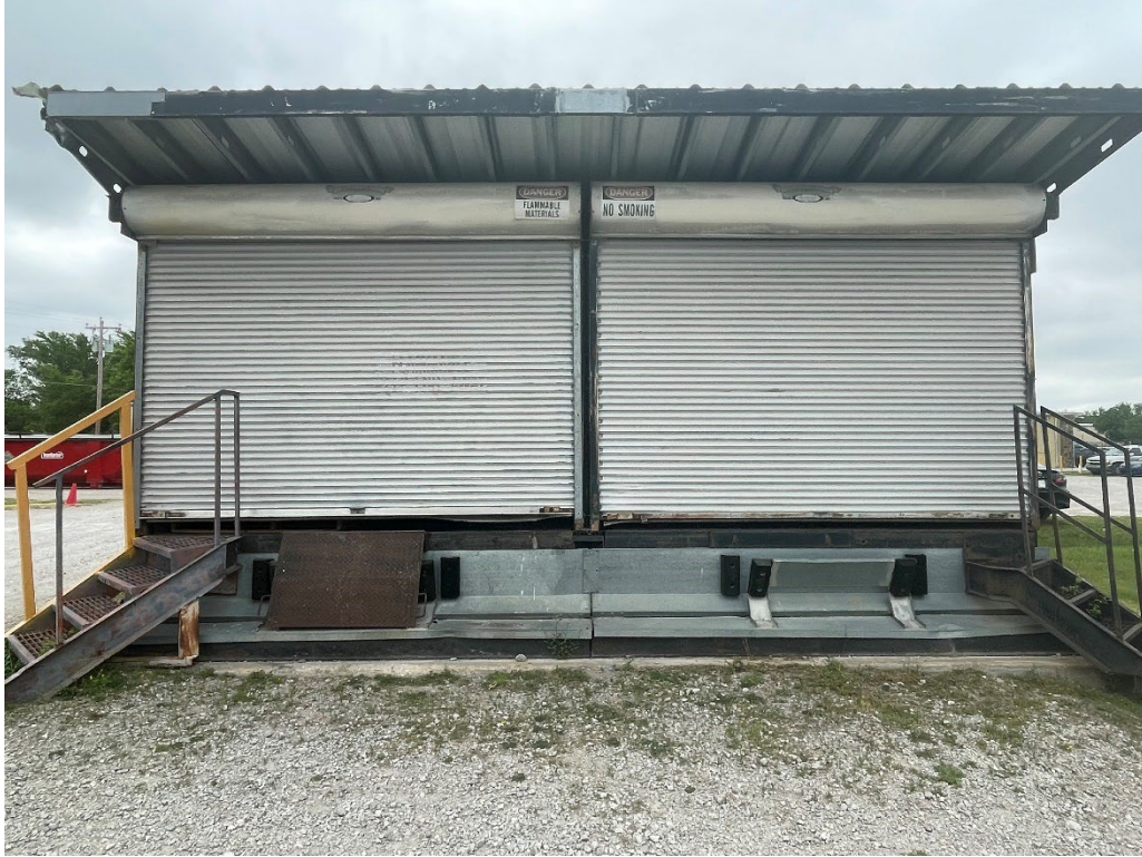
Figure 4: Metal Flammable Shelter
